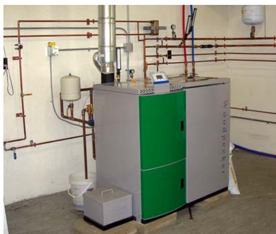
Fig. 1. Irish Woodpecker pellet boiler.
