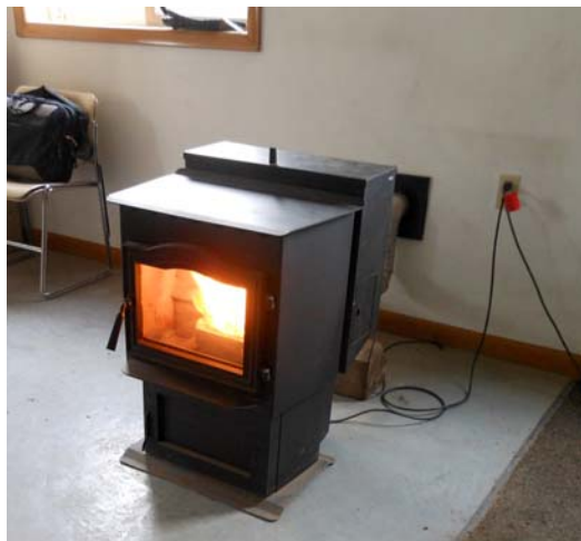
Fig. 1. Harman P43 pellet stove installed in the Town of Franklin highway garage.
