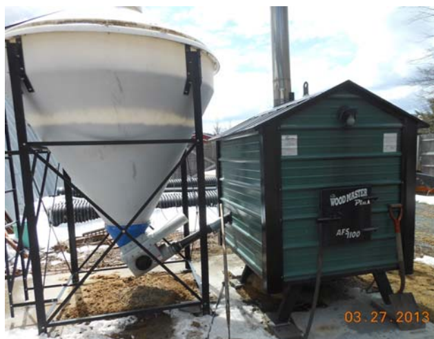
Fig. 1. Woodmaster AFS 1100 installed at the Town of Hunter highway garage.
