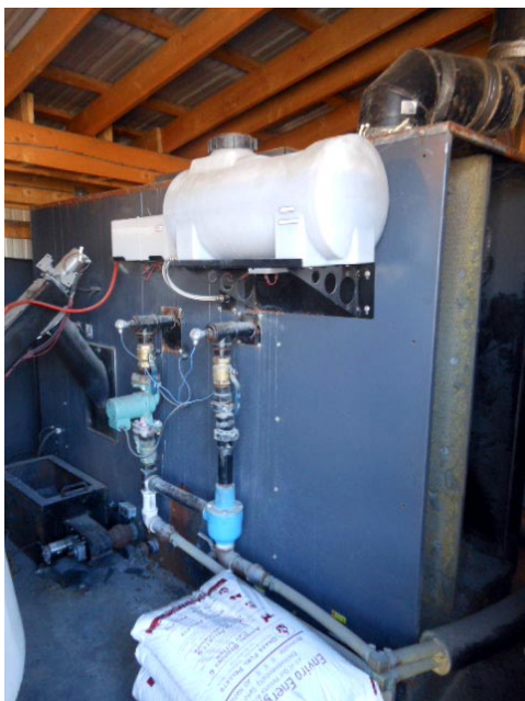
Fig. 1. LEI BB500 installed in the Town of Franklin highway garage.
